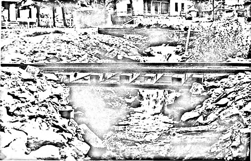
The replacing of a washed-out culvert at the lower end of Chase Gulch in Black Hawk by the simple expedient of a bed of rails is an example of make-do at minimal expense.
